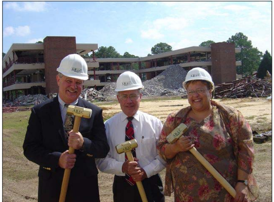
Interim President Tom Call, Director of Development Melvin Merrill, and Director of Student Life Bernice Hughes were among those who chipped the first bricks off Mitchell Hall as the demolition began last week.
