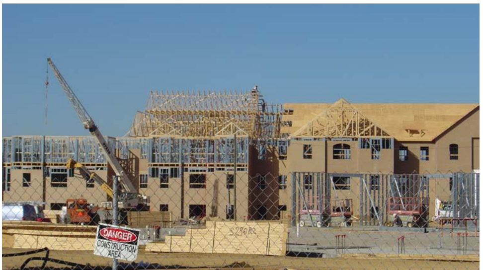
Construction continues on the new ABAC Place apartments. Tours of one completely furnished apartment will be available at 10:15 a.m. and noon on Saturday at the annual Fall Open Campus Day.
